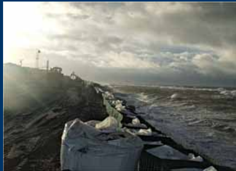
Sea wall damage September 4, 2007 Kivalena, Alaska
